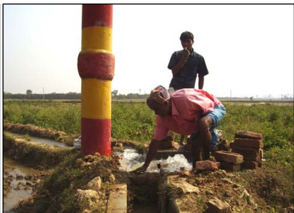
Underground Water Distribution Line
